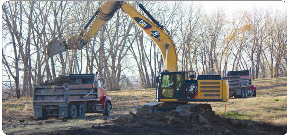
RECORD PHOTO BY JUSTIN LUSCHINSKI Construction crews were spotted stabilizing Grassmere Creek in West St. Paul for flood protection last week.
